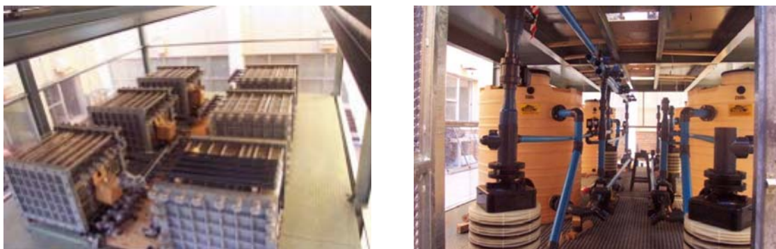
Figure 1 Typical VRB stacks and tanks (Courtesy Vantech)
