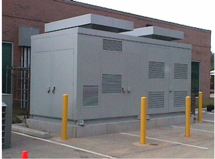
Figure 2-1 AEP's 500 kW (PQ) / 720 kWh (PS) NAS Unit
