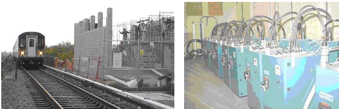
Figure 17 Flywheel Installation At NYCT Bay Equalizer Location, 10 1-MW Units In New Building
