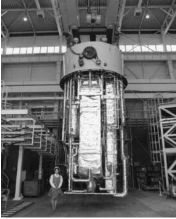
Figure 8 A large liquid helium refrigerator (JAERI)
