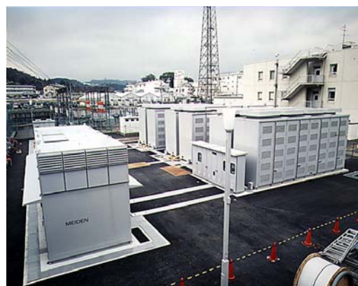
Figure 1-7. 6MW, 48MWh NAS System at TEPCO’s Ohito Substation
